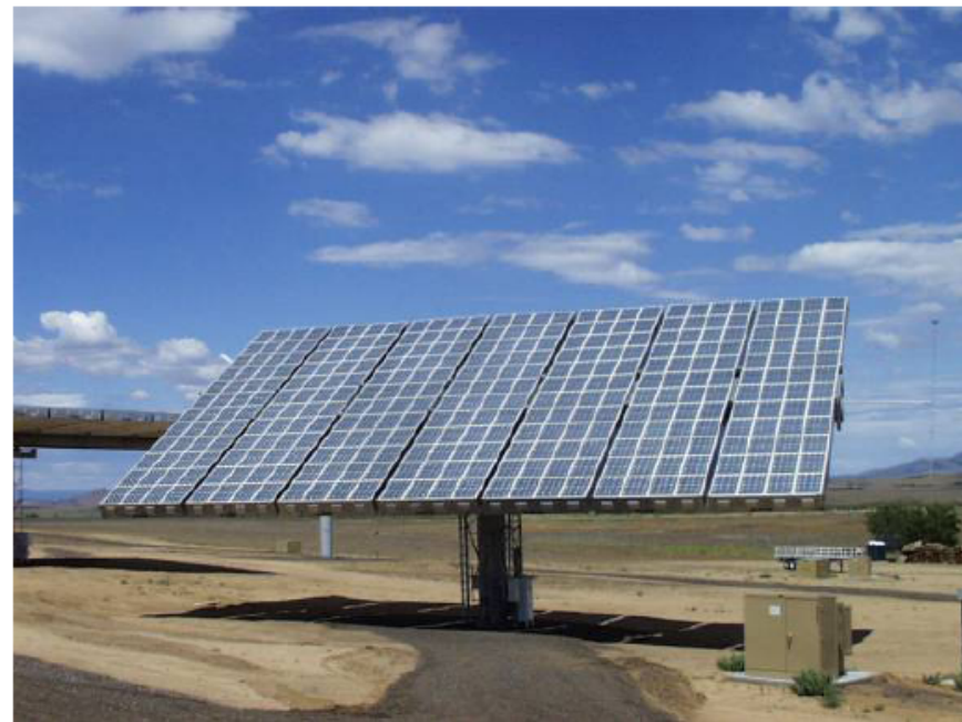
Arizona Public Service photo: Prescott 35 kW, single axis tracking system.
